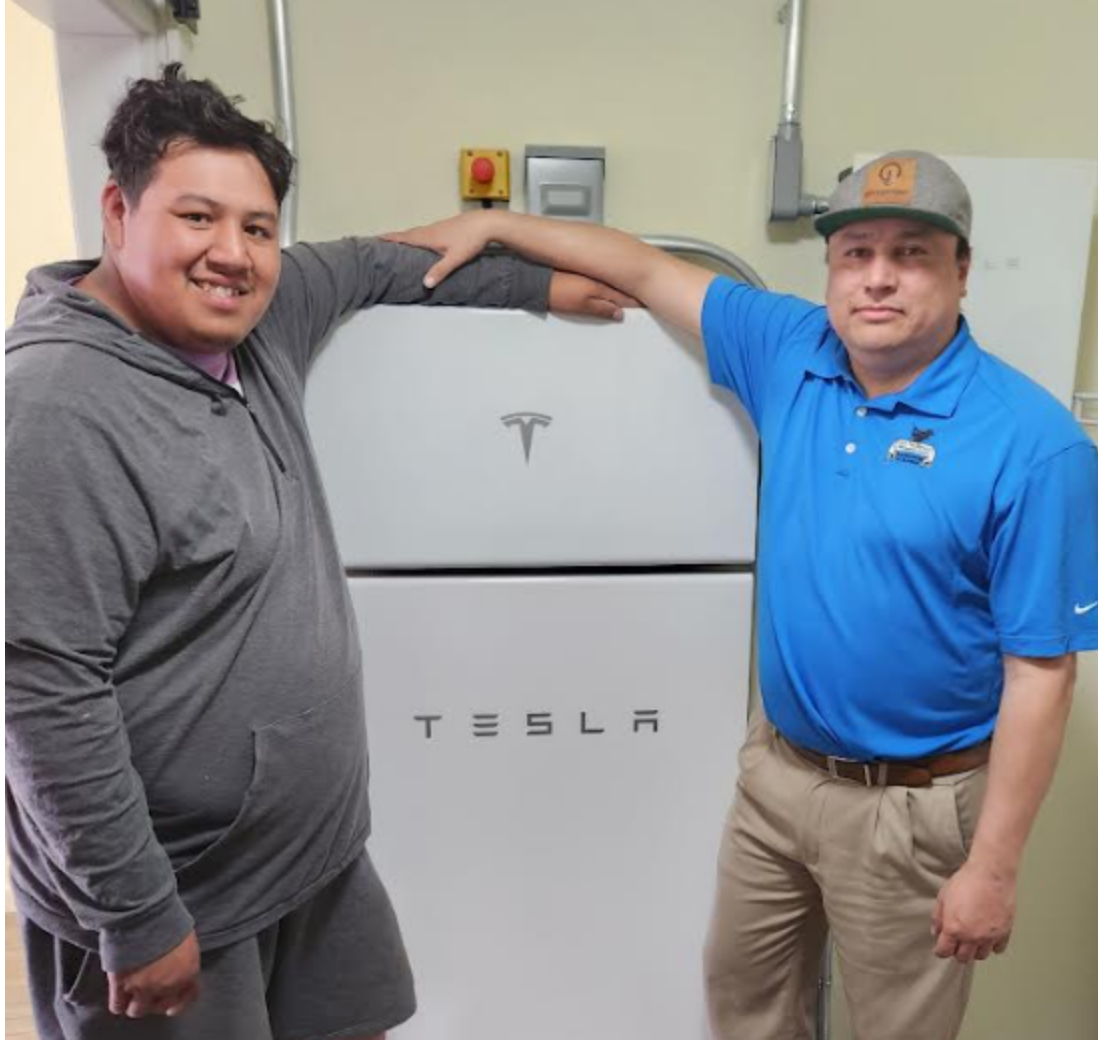
Daylon Fox (MHA Nation) proudly and Cody Two Bears (Standing Rock Sioux) present the installation of the first Tesla Powerwall in North Dakota as part of a solar+battery storage demonstration project in White Shield, ND
